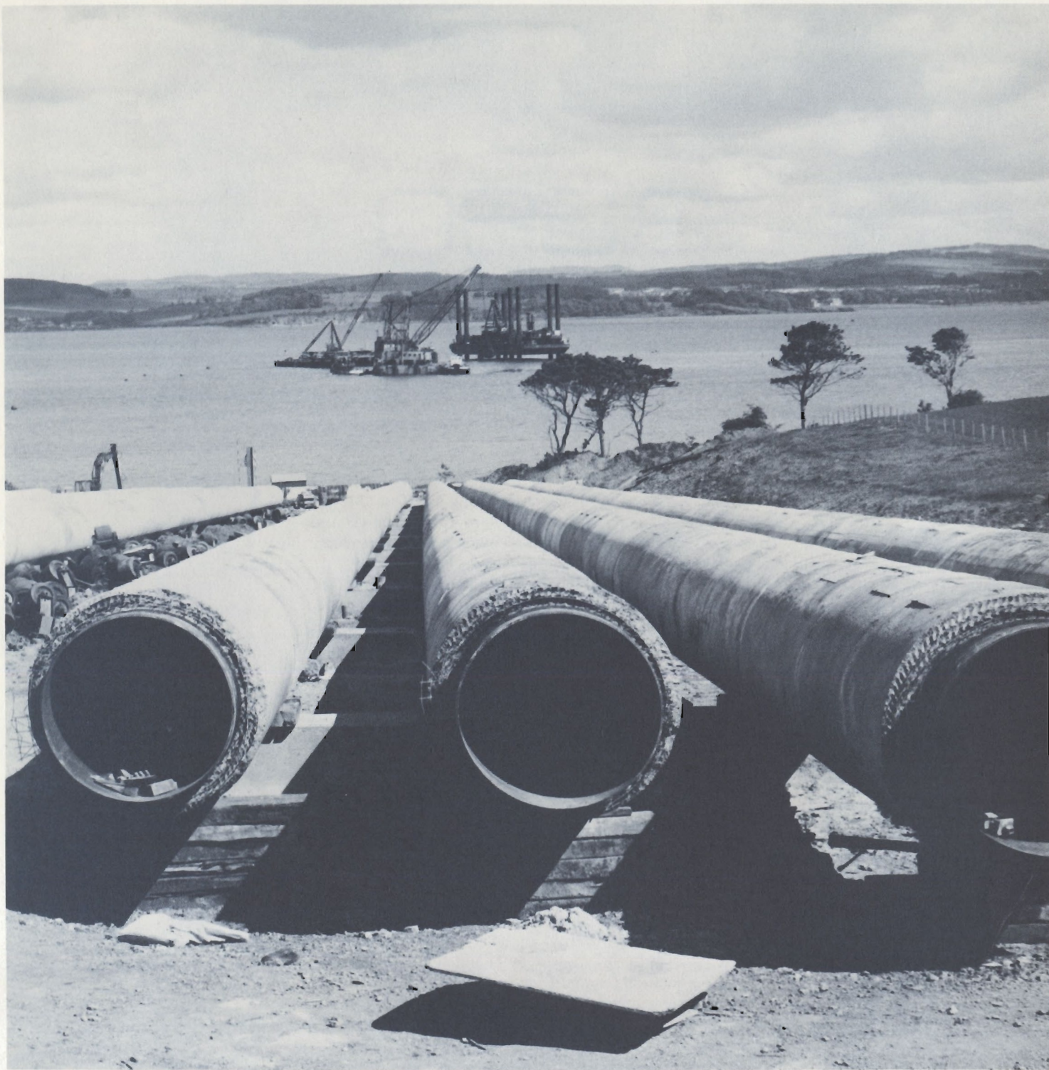
About ten fields in the North Sea off the coast of Scotland have now been proven for oil, while new discoveries continue. First deliveries are expected in 1975, with peak production by 1980. The scene here shows laying of pipeline in the Firth of Forth below the HP plant.
